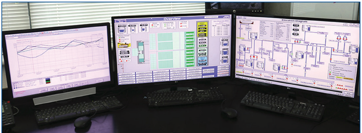
Supervisory Control and Data Acquisition (SCADA) system is the computer-based digital backbone of the District’s water system.
