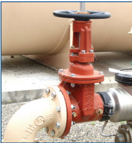
Replaced 40 broken valves in-house at a cost savings of roughly $5K per valve.
